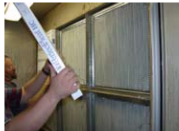
Specified Filters Prior to Test
